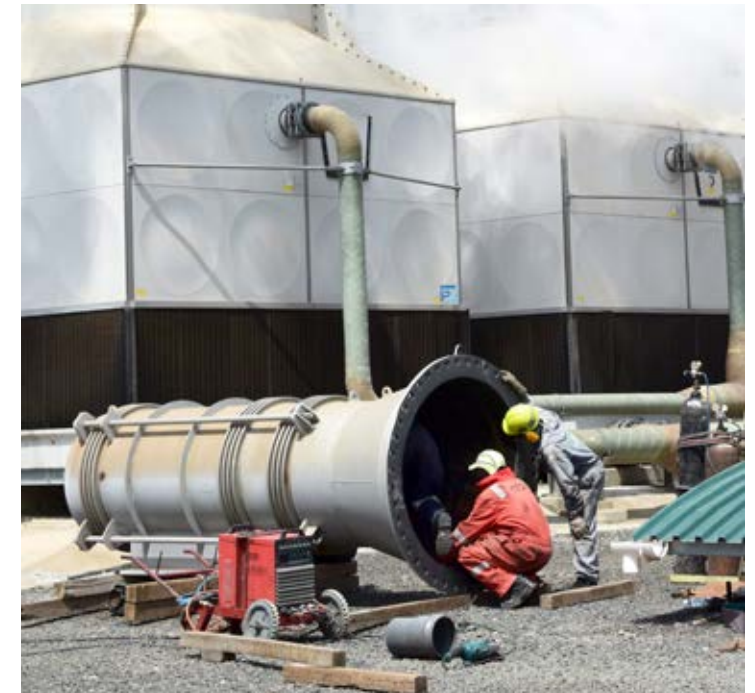
Olkaria geothermal complex and power station. All photos taken during the visit organized for the Global Geothermal Alliance Stakeholder Meeting in Nairobi, Kenya (June, 2015, IRENA)
