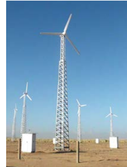
1 MW Hybrid electrification project (Wind, Solar PV & Hydropower) will provide clean and reliable energy to 165 small rural villages (selected for funding in the IRENA/ADFD Project facility)
