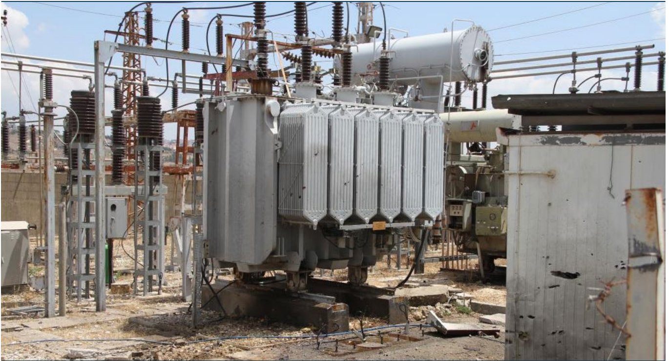
Figure 1. Power station damaged by an Israeli strike in Marjaayoun
