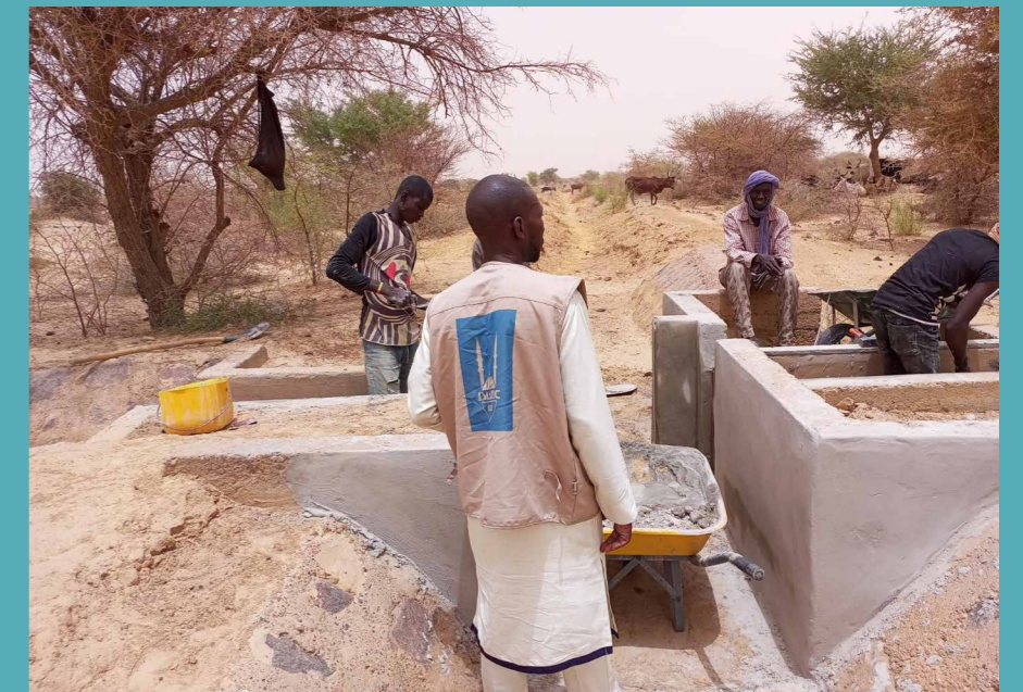
Islamic Relief supervises a water trough being constructed in Tourchawane village, Gourma-Rharous, Mali.
