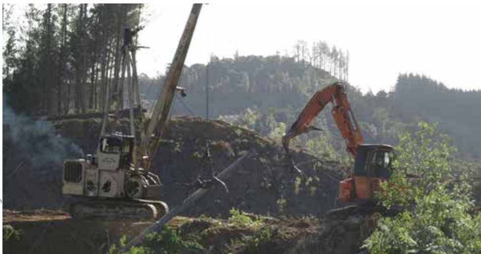
PHOTO 29 Work at a landing with many opportunities for things to go wrong
