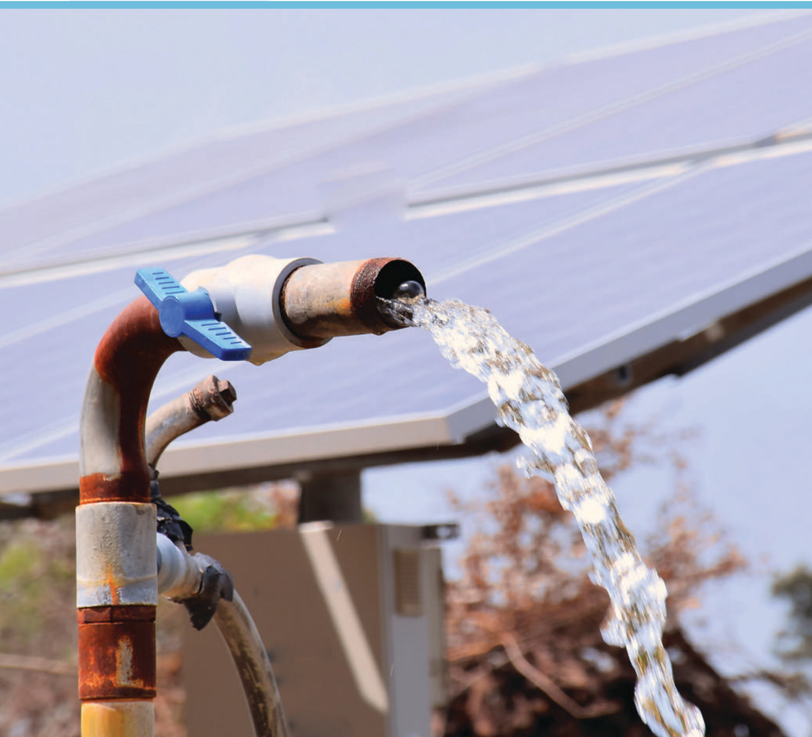
Equipment for a solar-based irrigation project.
