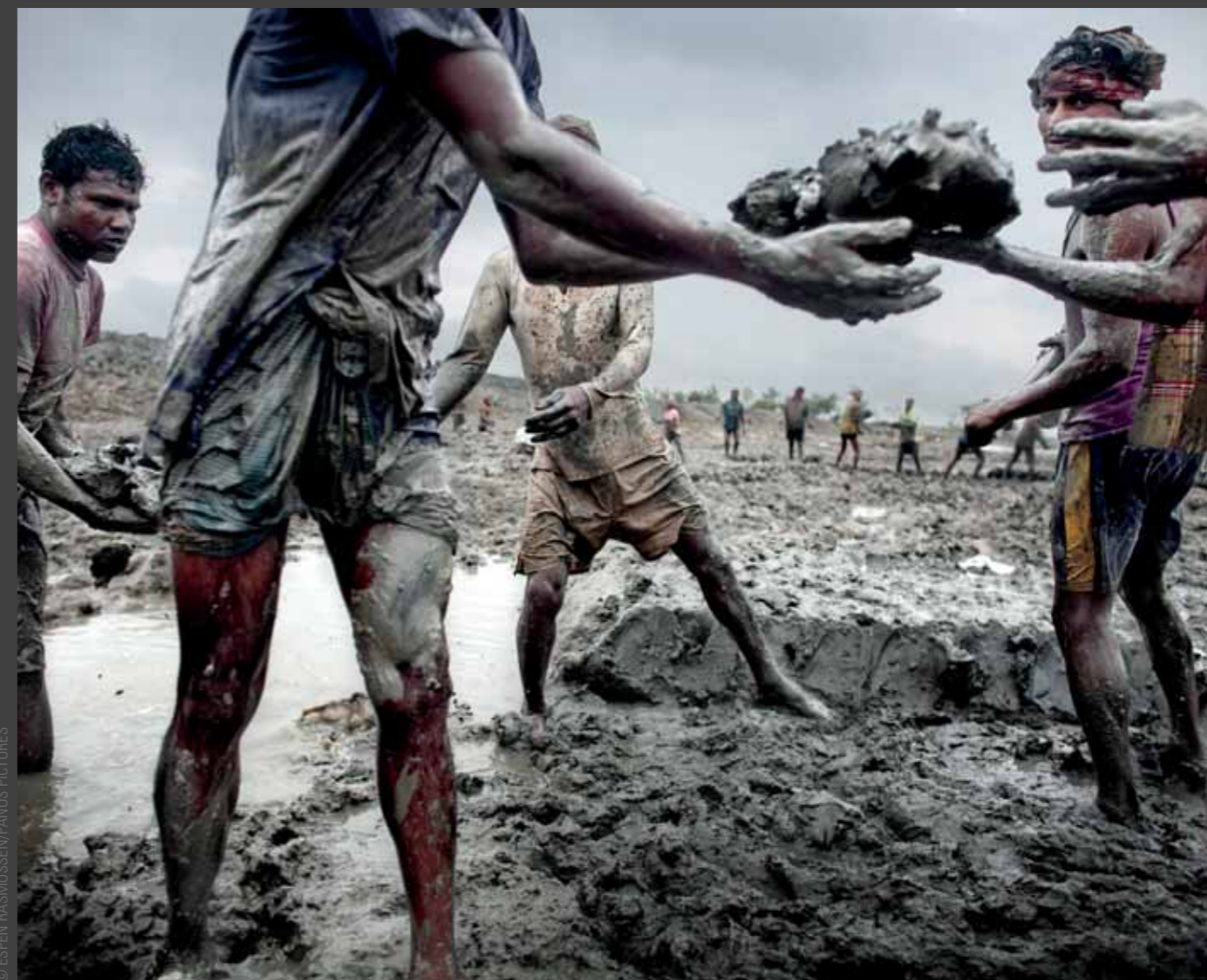
Local people in Padma Pakur, Khulna Division, form a human chain to build a new flood barrier after Cyclone Aila in 2009.
